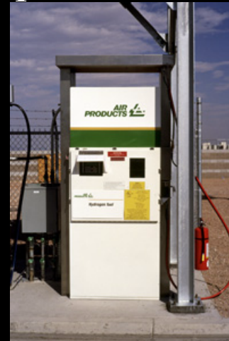
Hydrogen fueling dispenser at the Las Vegas Energy Station - Air Products and Chemicals, Inc.
